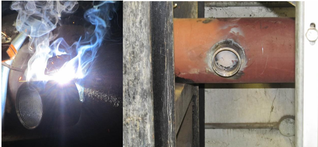
Above: A 2"/50mm Threaded short is welded to the outside wall of existing pipe work
