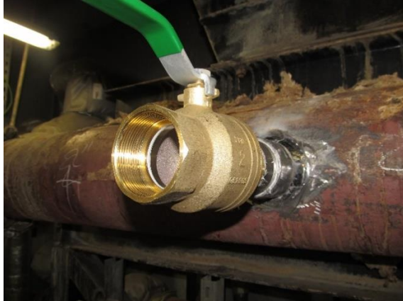
Above: A new 2" isolating ball valve is fitted to the new threaded short
